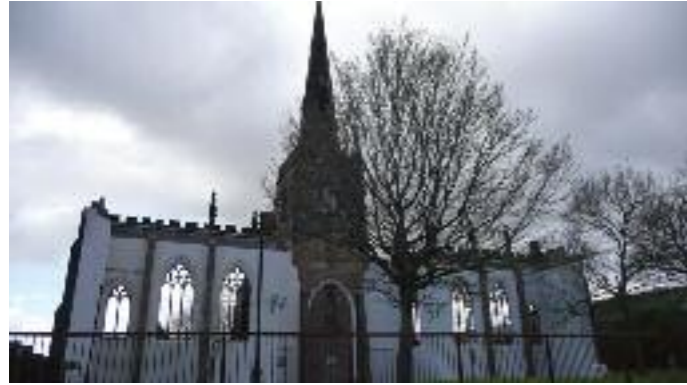
The original inside wall of St. Mary's church has now been rendered
